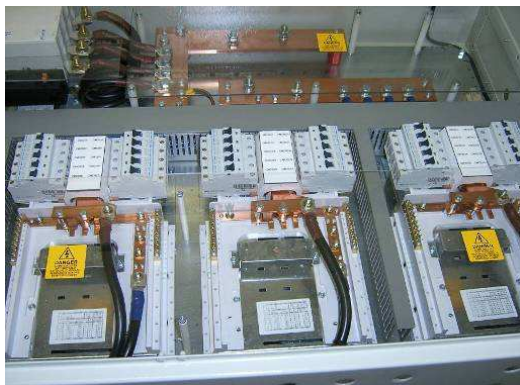
Typical pitch-side junction box
